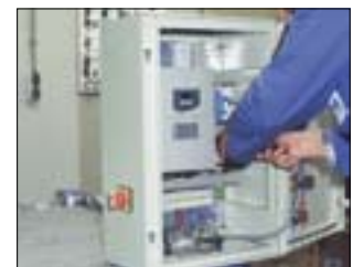
Controle paneel met frequentie omzetter Control panel with frequency inverter
